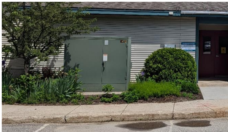
Figure 15 6 Spruce St. Electrical Distribution Transformer
